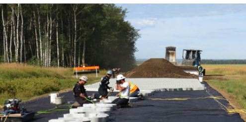
(top) Detail of crushed gravel top course (bottom) Tough Cell crew deploys ahead of infill
