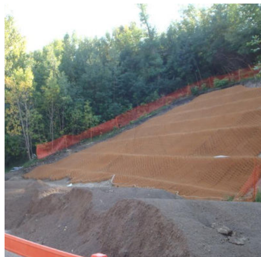
Tough Cell ® installed
