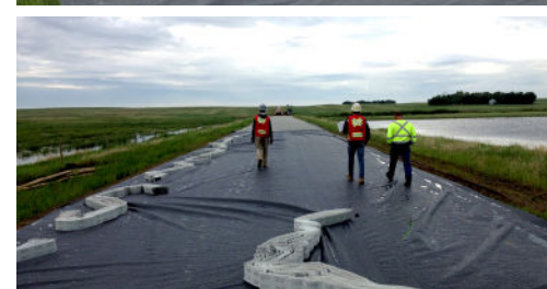
(top) Installation of geotextile to ground (bottom) Tough Cell® preparing to be stretched
