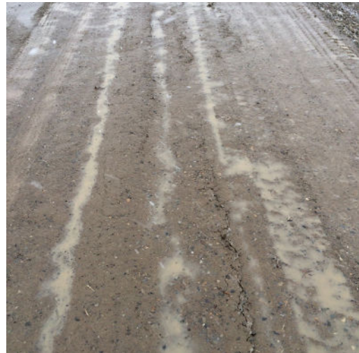
Water issues from heavy rain and high water table prior to Tough Cell® installation
