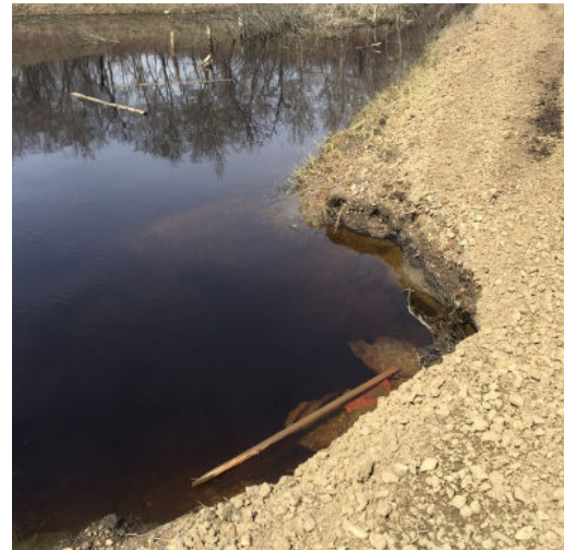
Loss of road material into surrounding water
