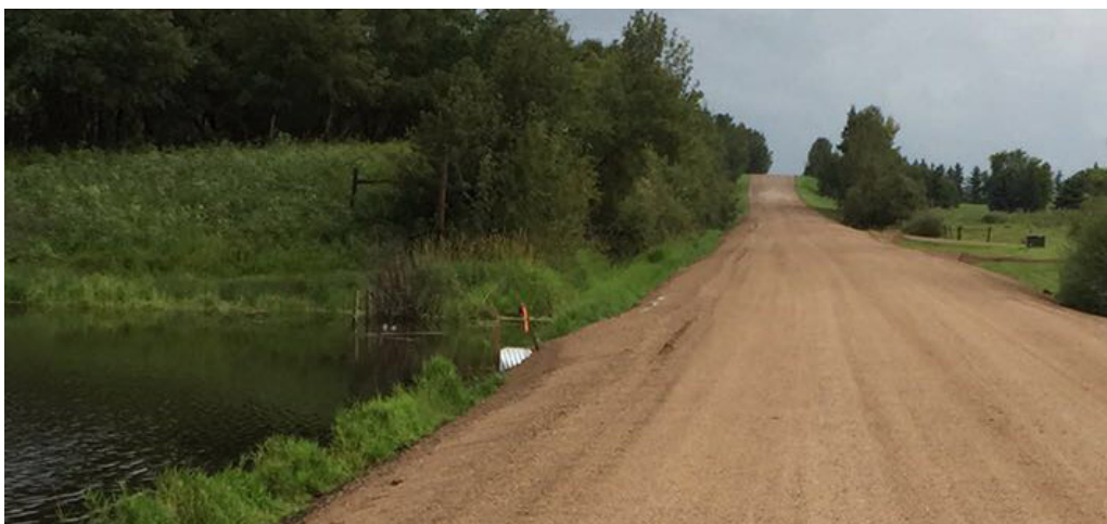
Roadway 2 weeks after completion, following 2in. of rainfall and resumption of heavy traffic.
