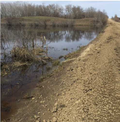
Encroachment of water to roadway
