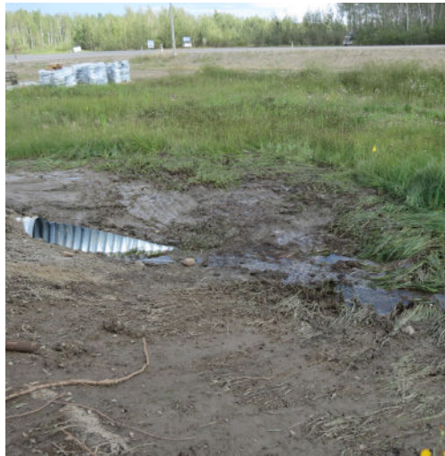
Mud and drainage issues before construction
