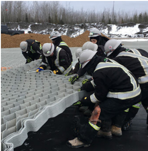
Tough Cell® installed
